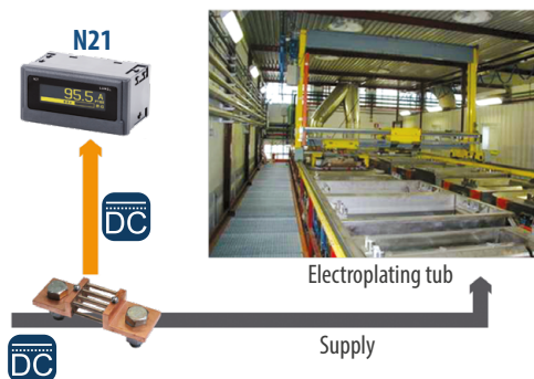
CURRENT MEASUREMENT IN AN ELECTROPLATING PLANT
